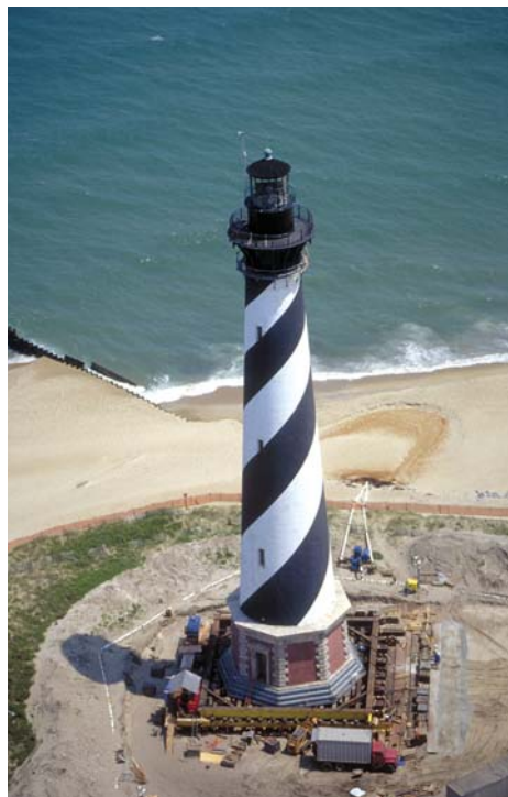
The Cape Hatteras lighthouse being prepared to be moved to keep it above the rising sea.
